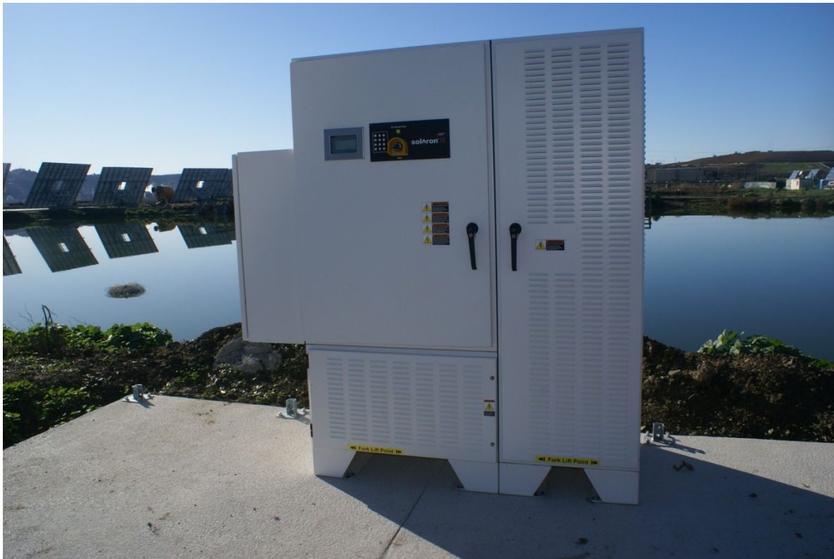
Solaron 250kW Inverter
